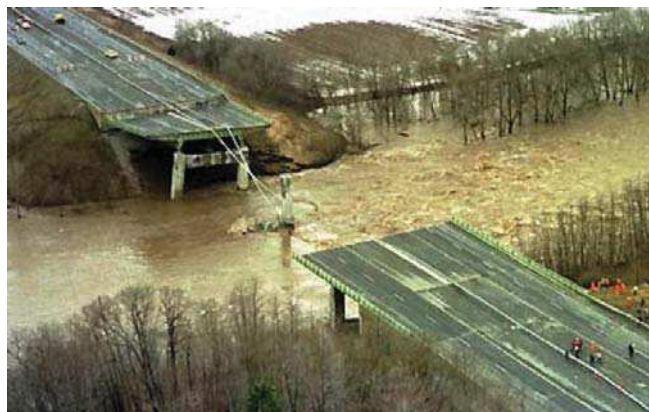
Figure 1. Example of a highly dynamic environment ideal for ASV deployment for the task of infrastructure inspection.
